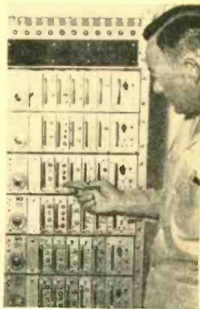
Banks of signal processors are part of automatic head-end operation. Devices amplify signals and sometimes switch channel frequencies.
